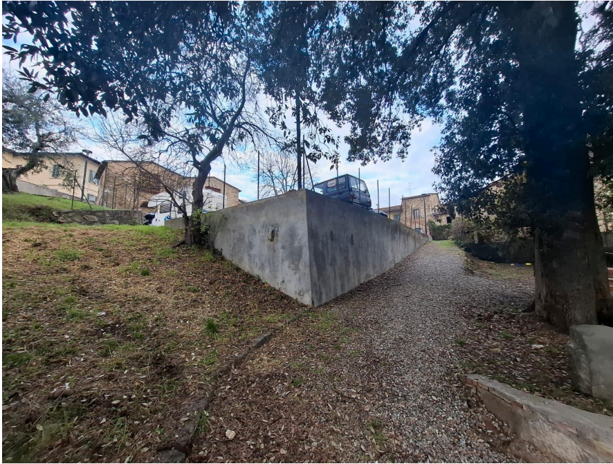
Fig 18 - Lack of stairs
